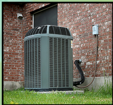
Electric Heat Pumps
