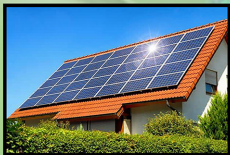
Roof Top Solar Panels
