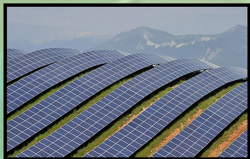
Solar Arrays communal energy meters at each building
