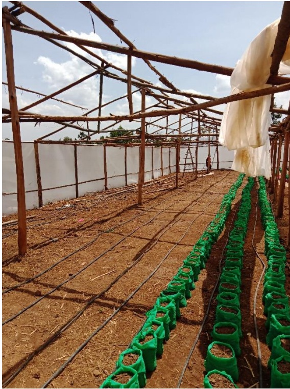
This photo illustrates how the framework for the greenhouses is constructed using local wood.
