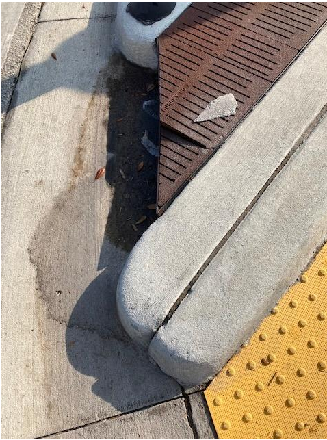
03.13.23 Damaged grate at Main/S 7 th St – repaired 3.14.23
