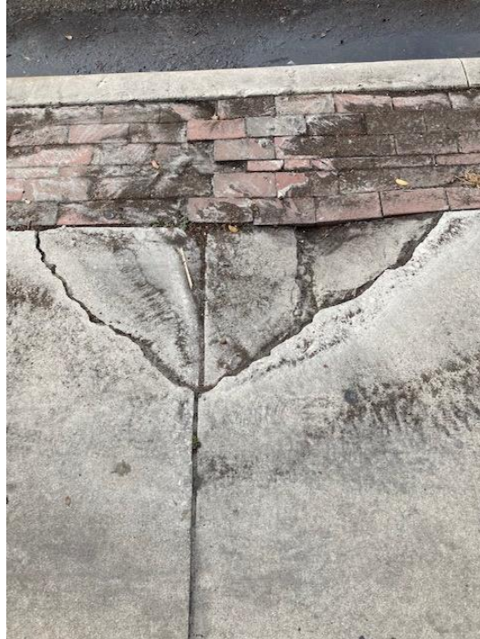
04.10.23 damaged sidewalk was reported for repair
