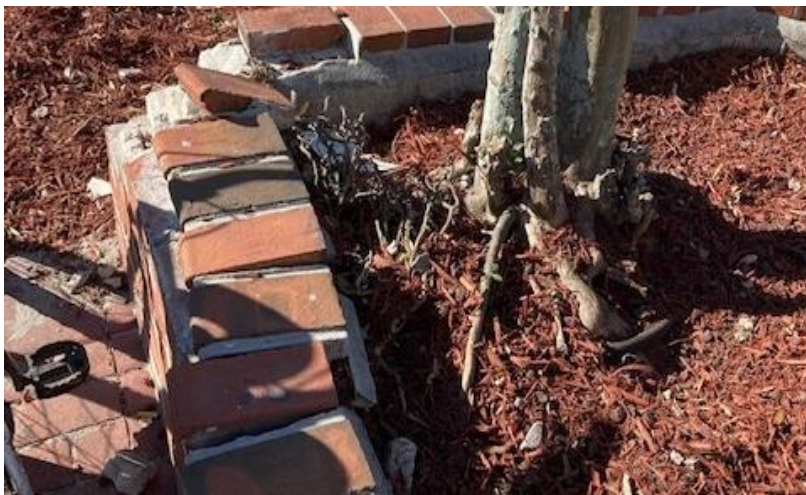
02.13.23 damaged bulbout planters N 3 rd St
