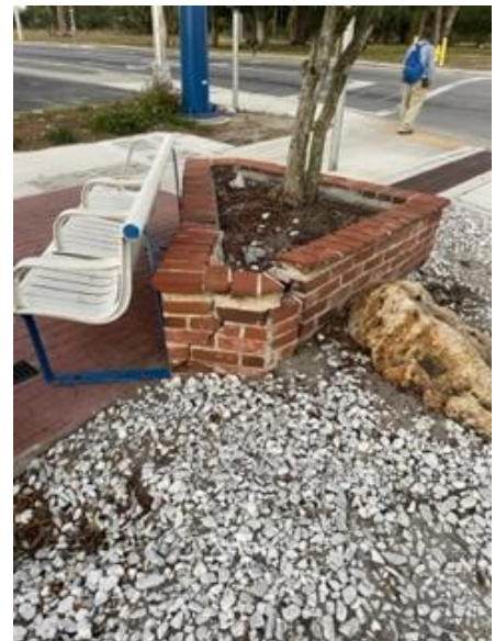
02.13.23 damaged bulbout S 9 th St
