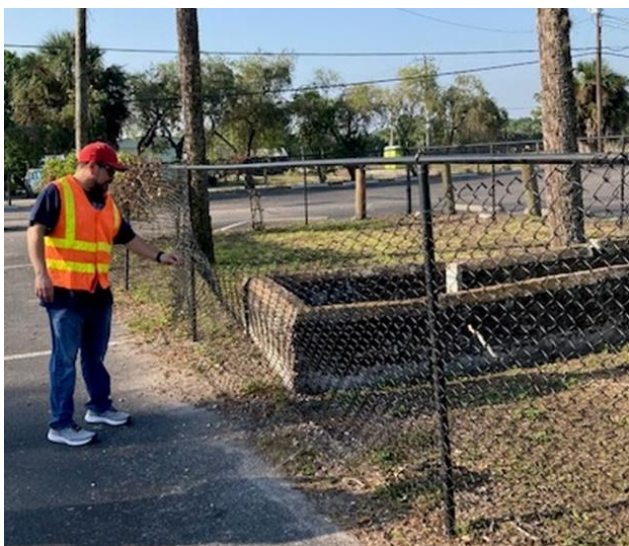
03.13.23 P&R requested to repair the chain linked fence
