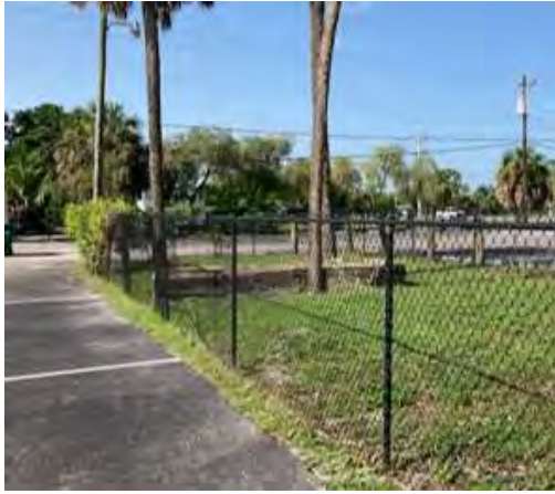
07.10.23 Fence line sagging
