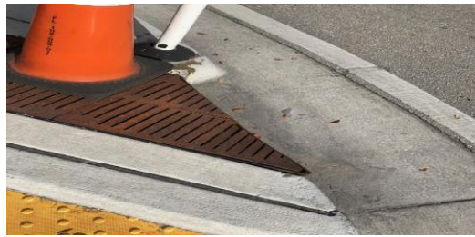
1.10.22 newly repaired grate has a crack near tip
