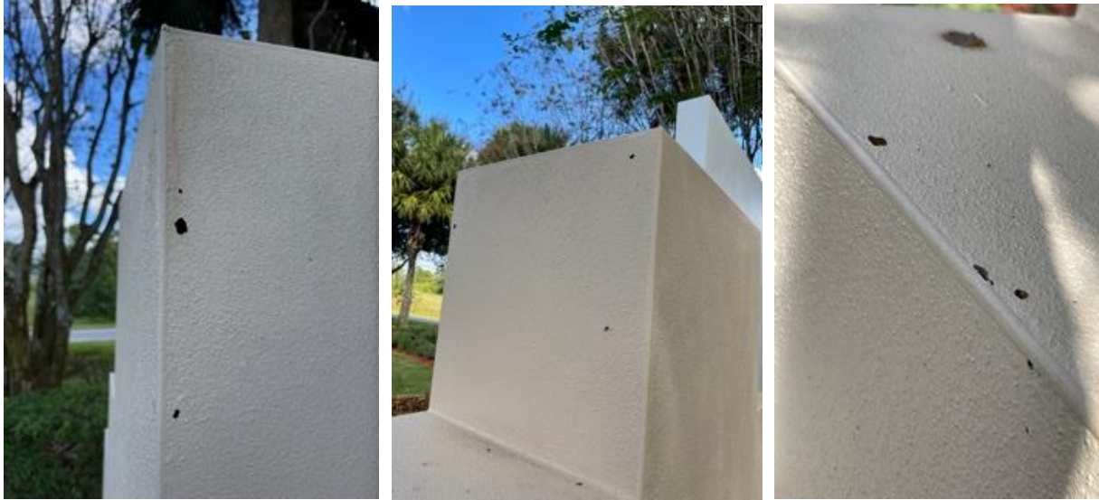
Stucco Failure at Triangle Monument 11.16.21
