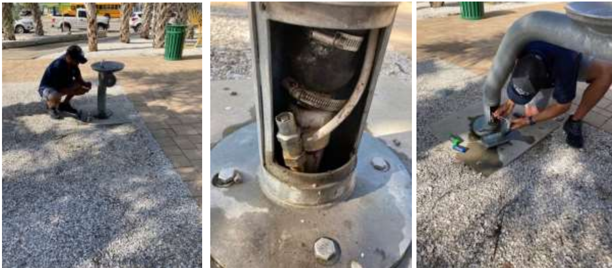
06.13.22 Fountain Leak needs repairs
