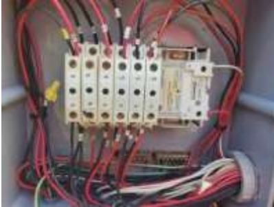
05.10.22 Contactor needs replaced
