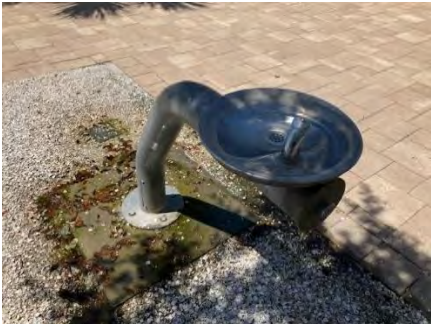
05.01.24 Requested Work Order to repair leak.
