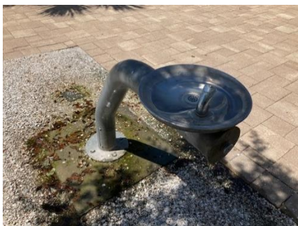
05.01.24 Requested Work Order to repair leak.
