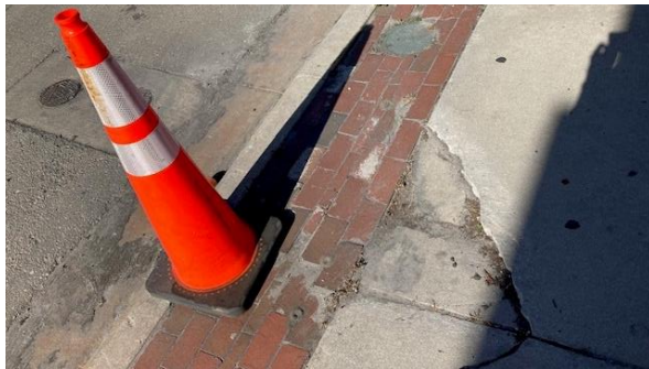
03.13.23 Leaning Pole N 9 th – repaired 3.14.23
