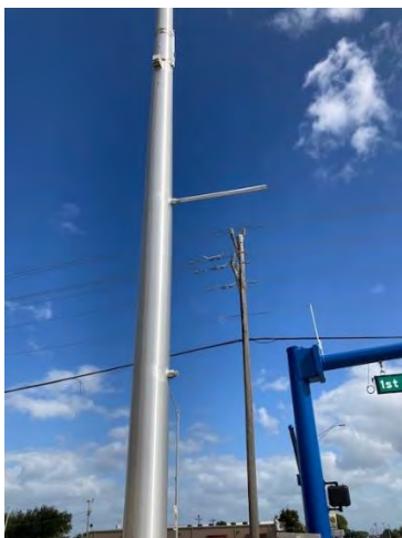
Pole 22 at Zocalo Plaza missing banner arm
