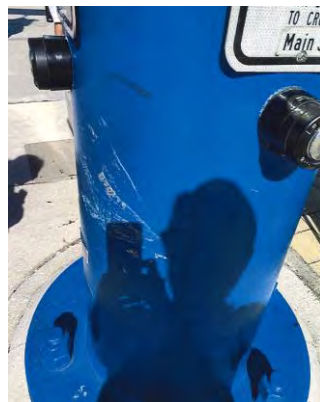
09.16.22 damaged mast arm pole
