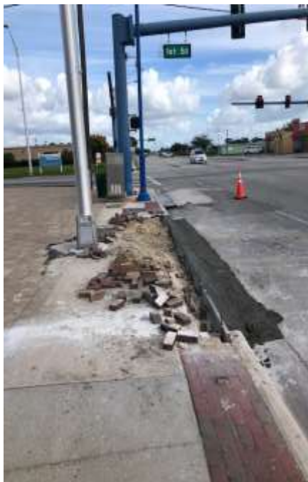
FDOT replaced the concrete curbing from the installation of the new light pole at Zocalo on November 6, 2020.
