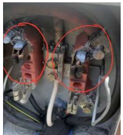
07.14.22 damaged meter identified by Simmonds
