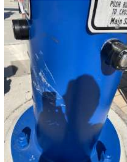
09.12.22 damage to mast pole
