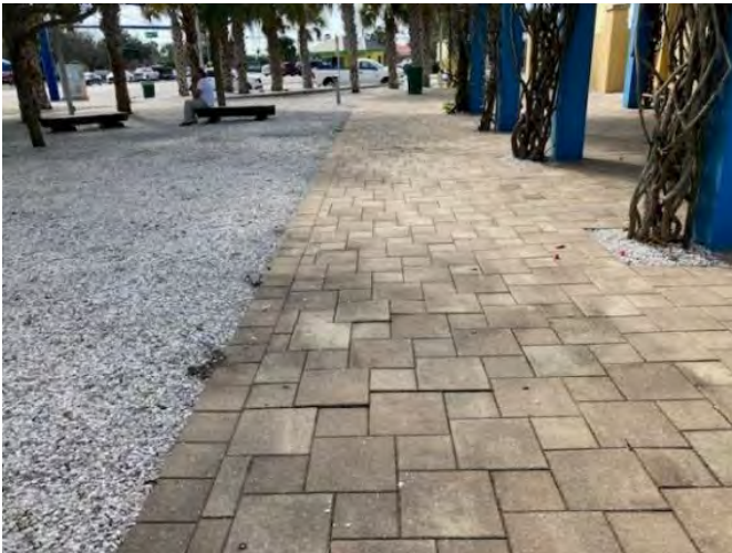
5.30.23 before trip hazards were addressed
