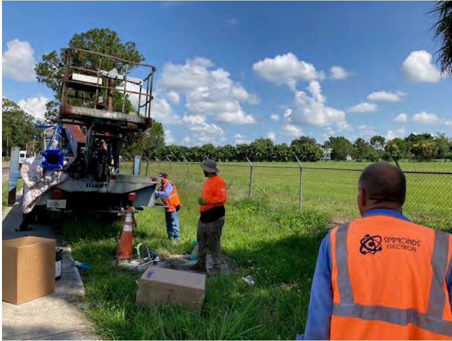
07.06.23 Installation of Pole #20 on the curve N 15 th St south of Roberts Ave
