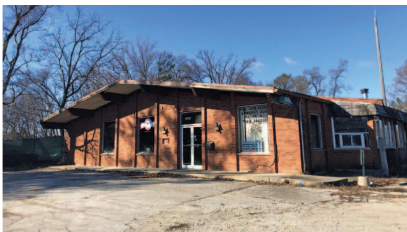
A staple of Winfield's business district for decades, Winfield Fuel and Material is being demolished and the site prepared for a luxury apartment community.
