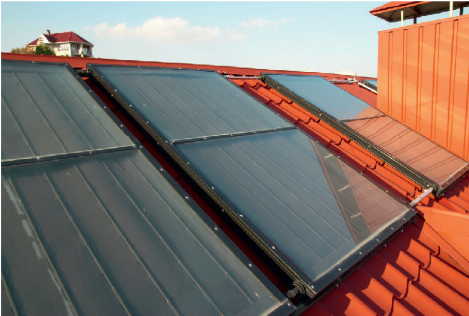
Figure 2.3 Photo of a solar hot water panel.
