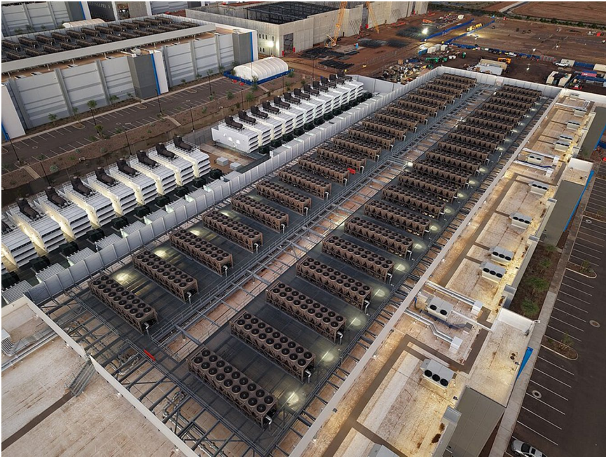
Roof of a data center featuring cooling towers and backup generators in Mesa, Arizona.
