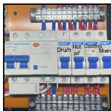
NEW CIRCUIT BREAKER SYSTEM
