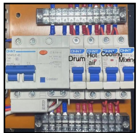
NEW CIRCUIT BREAKER SYSTEM
