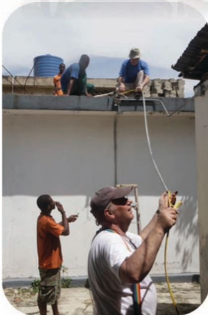
John Morgan and John Messina running a new power line at St. Pierre clinic.
