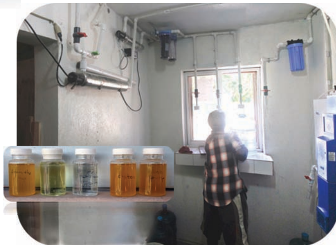
Water purification systems at the orphanage and retail window. Insert: Results of purification tests. Water sold is excellent quality (middle bottle).
